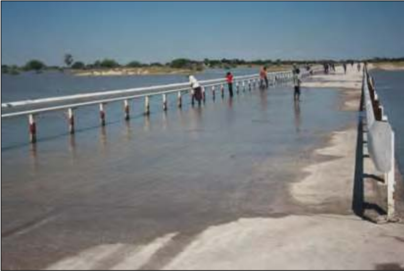
Picture 7 Water over the Bridge along the Oshakati – Ompundja road
