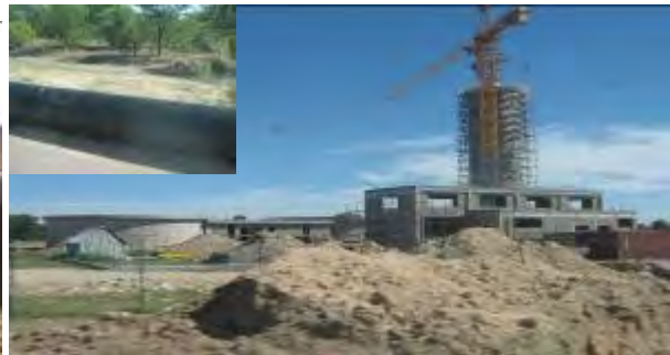
The water Treatment plant in Xangongo that will supply water to southern Angola, and the pipeline in the insert
